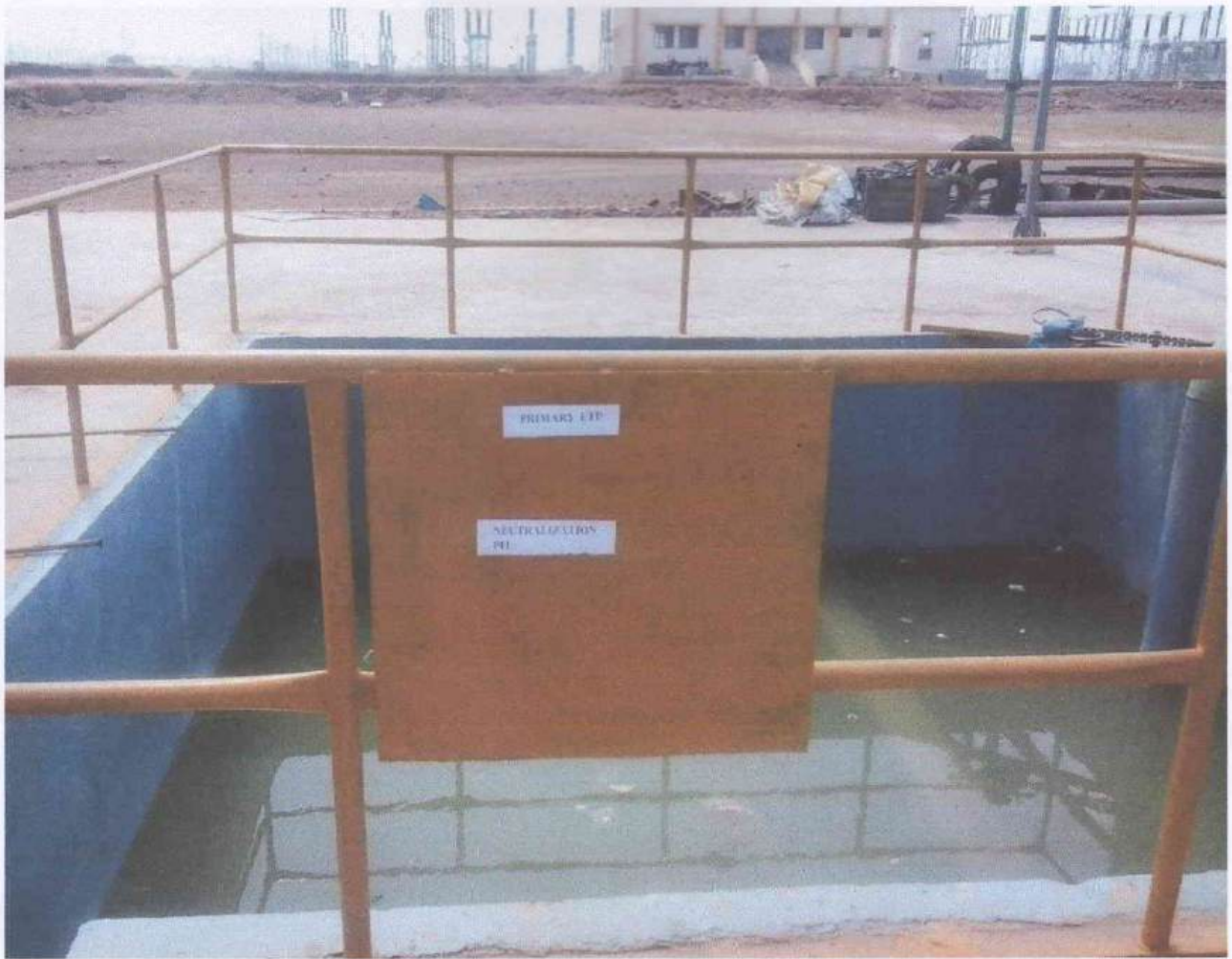
Photo of Neutralization Pit
